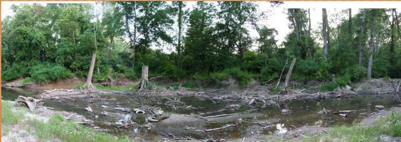
Address severe stream bank erosion
