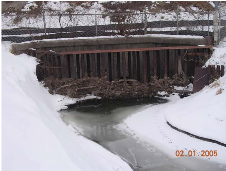
Photograph No. 25 Orientation: North Description: Otter Creek at Willow Cemetery, north of Pickle Road; note debris trapped at entrance to tunnel going beneath Sunoco property Location: Otter Creek (14) Date: February 2, 2005
