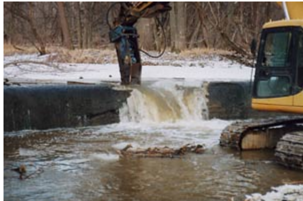
Removal of the Camp Miakonda Dam on the Ottawa River in December 2002.
