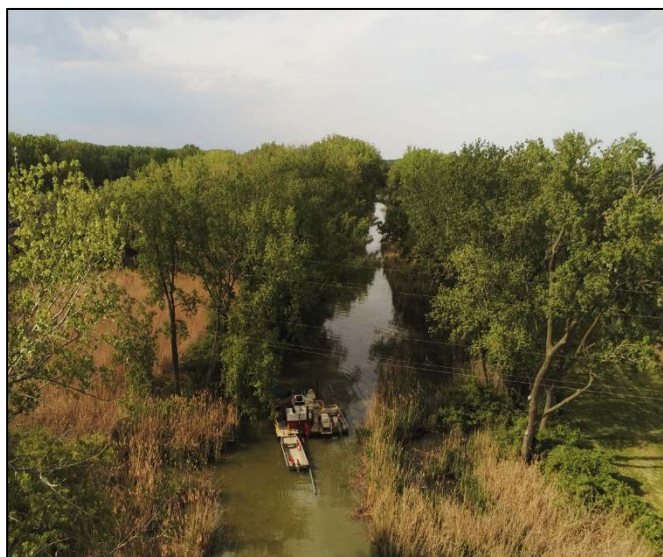
Figure 29. Dredging operations at the confluence of Otter Creek and Maumee Bay in Summer 2021. Photo from: US Army Corps of Engineers
