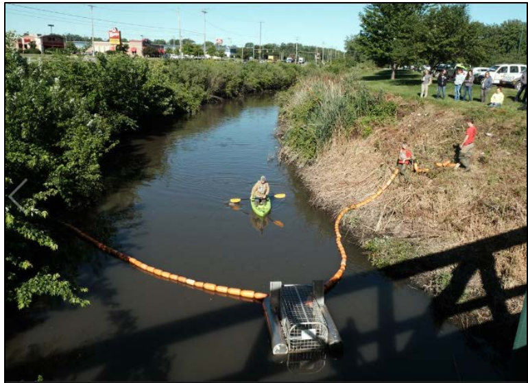
Figure 16. Installing trash capture device in Shantee Creek on June 22, 2021. Courtesy of The Blade.
