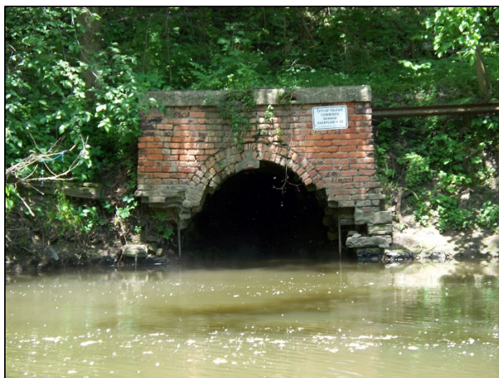
Figure 4. CSO outfall along Swan Creek, 2008 Photo by: Cherie Blair
