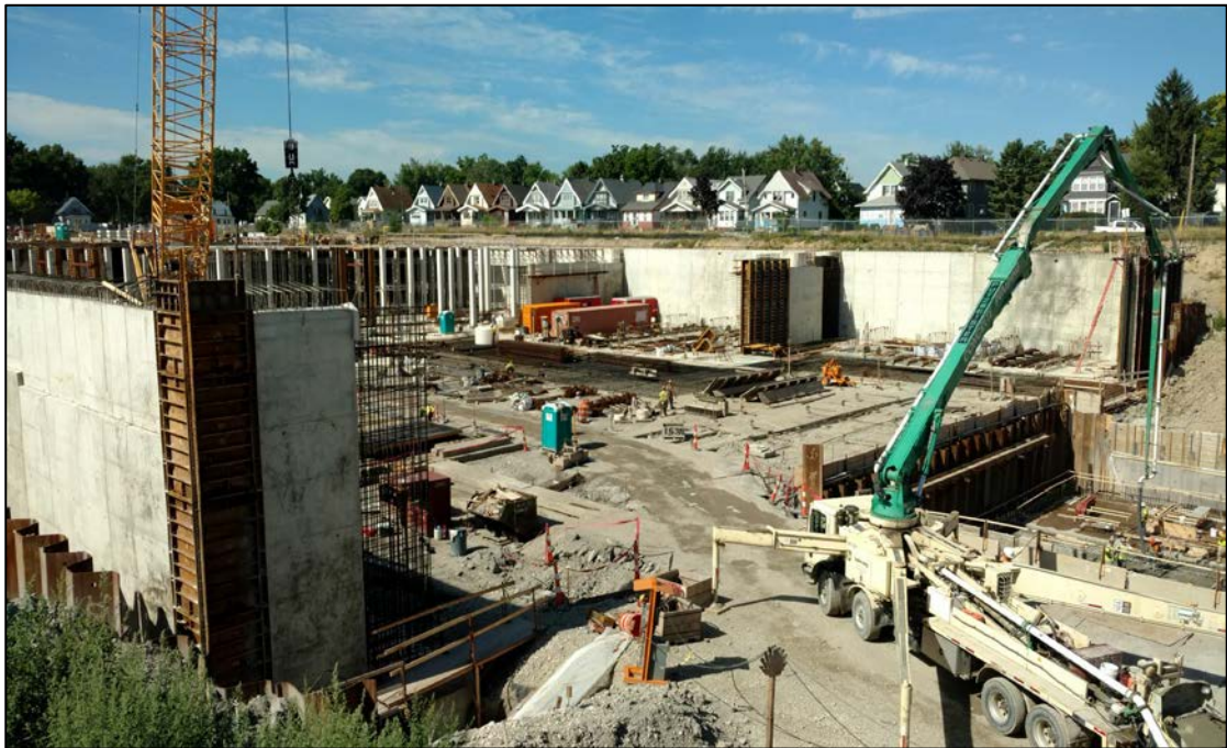
Figure 8. Joe E. Brown Park Ottawa River south CSO storage basin under construction. Construction completed in June 2018.
