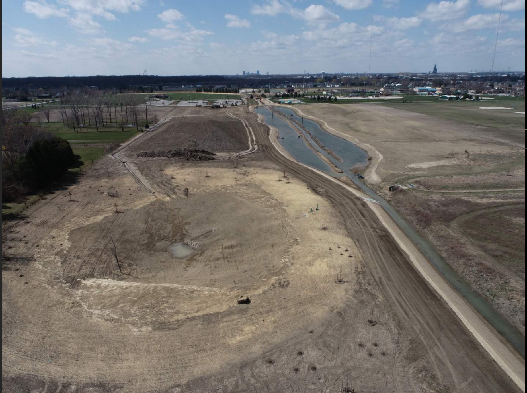
Constructed Wetland (South Side), Wolf Creek Stream and Floodplain Restoration Project, March 2024
