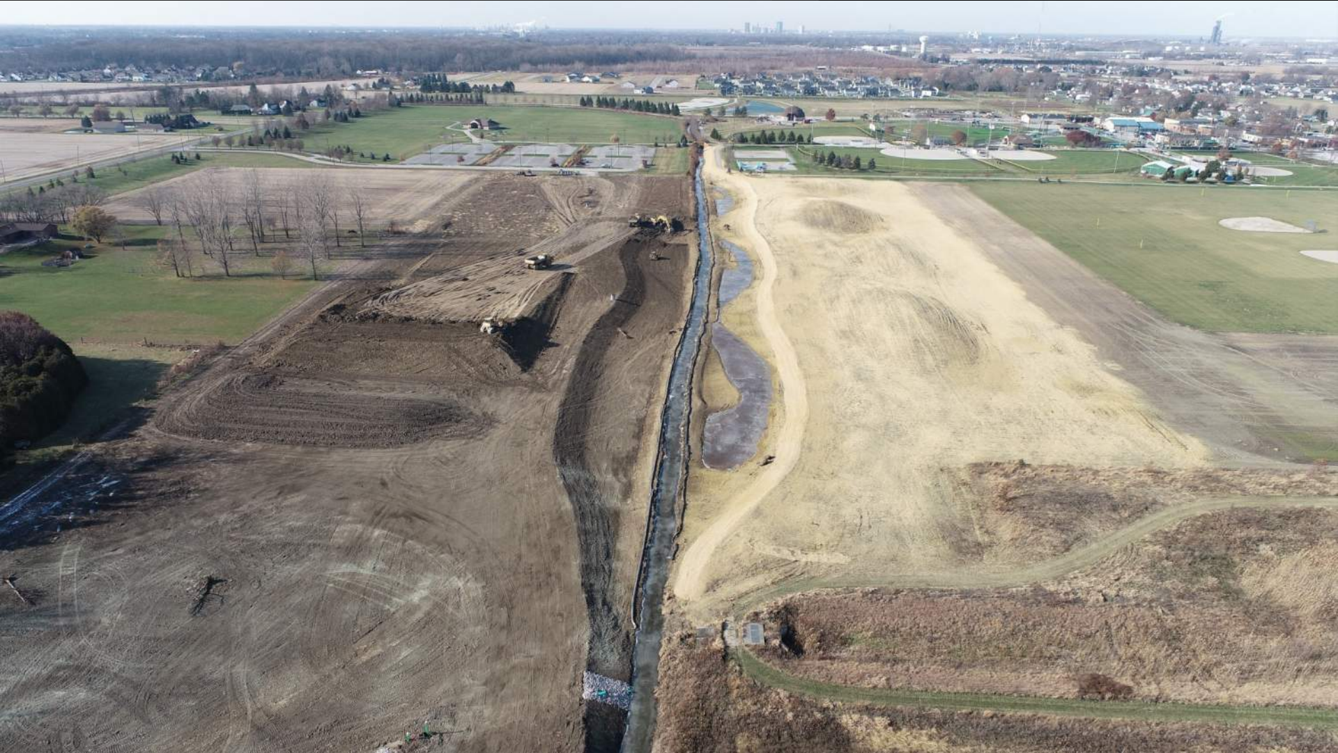
Construction of South Floodplain, Wolf Creek Stream and Floodplain Restoration Project, December 2023
