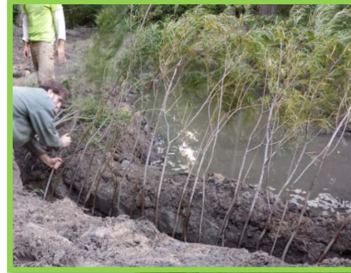
After LPSTP is placed, some soil is added to cover the LPSTP, and then live poles are installed over the LPSTP (parallel to the body of water).
