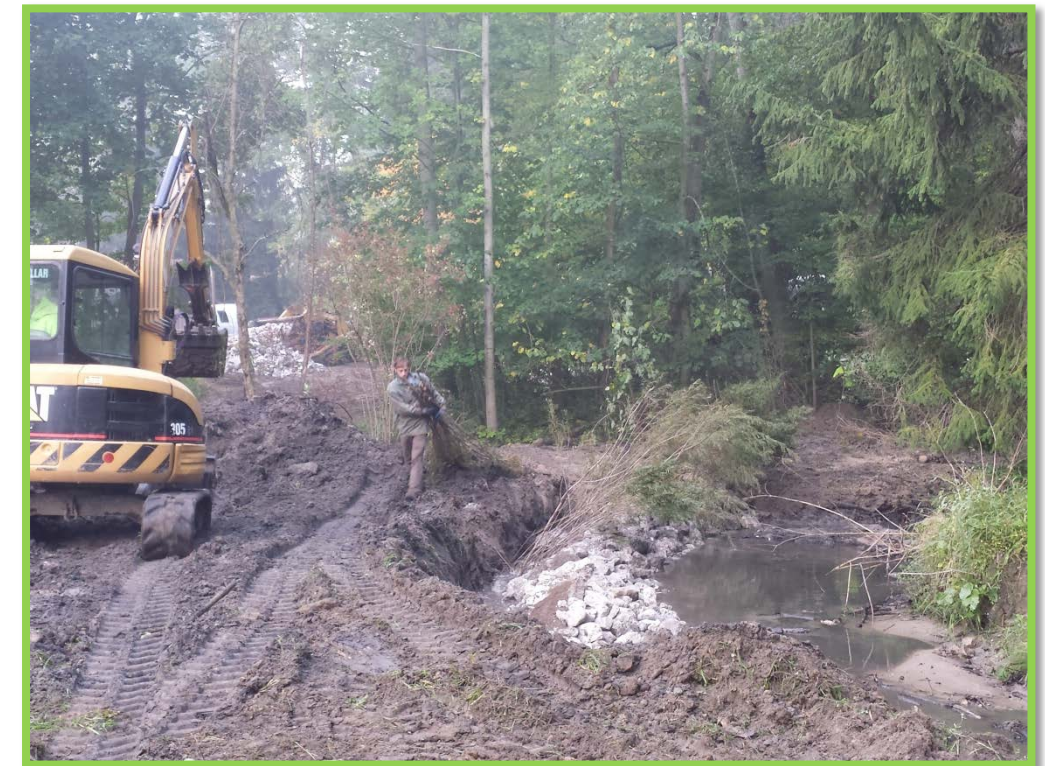
Image 2: Crews install Live Siltation at Camp Miakonda, Hartman Ditch, Sylvania, OH. Kyle Spicer.
