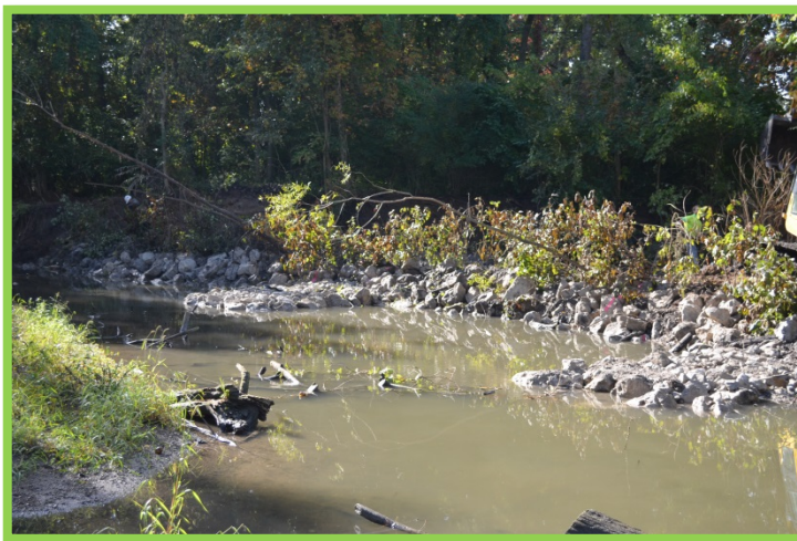
Image 1: Live Siltation installed over Longitudinal Peaked Stone Toe Protection at Camp Miakonda, Ottawa River. Kyle Spicer
